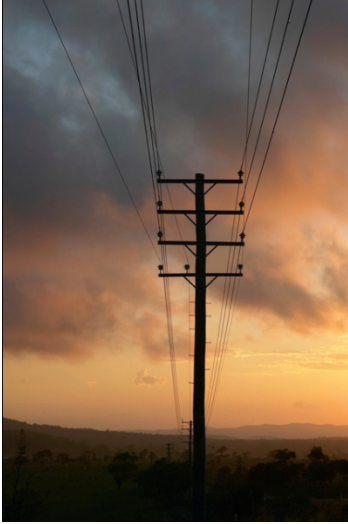
Figure 1: Telephone pole on the PSTN
